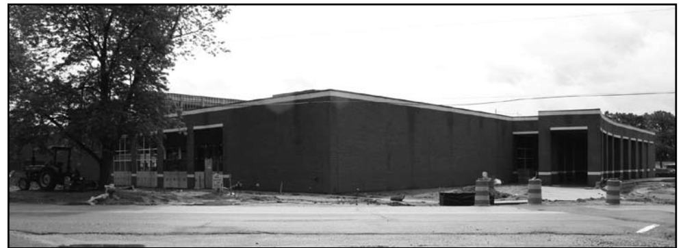
Seawater Research Lab: This 46,000-square-foot building, which will house numerous flow-through tanks for culturing fish, shellfish, and sea turtles, is currently on schedule with completion slated for February 2007. Crews are currently grading the site and installing sidewalks, and will begin installing the roof in July. The interior and exterior (brick) walls are complete and window installation is in progress. Interior mechanical, plumbing, and electrical work is underway. A separate Water Treatment Building (not shown) is nearly complete.
