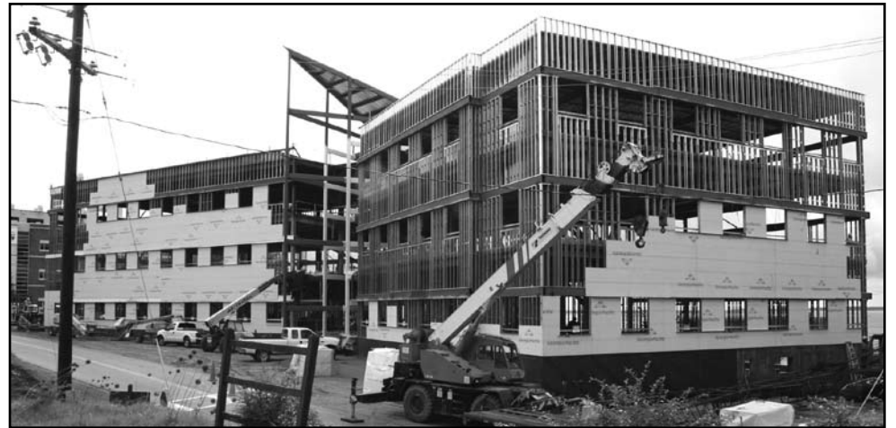
Andrews Hall: This 71,000-square-foot research facility is currently on schedule with completion slated for February 2007. The structural steel is in place and 90% of the concrete floors have been poured. Crews have begun framing exterior and interior walls, and will soon begin to install the roof, exterior brick walls, and windows. Interior mechanical, plumbing, and electrical work is underway and installation of the rooftop HVAC units is scheduled for the last week of June.
