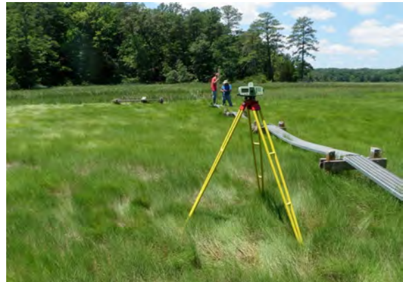
Figure 8.1. Establishing vertical control of monitoring infrastructure along a saltmarsh transect. Image credit: W. Reay.
