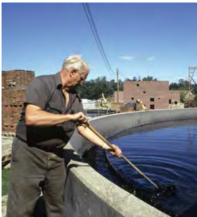
Cleaning the sludge thickener tank at the Water Pollution Control Plant, Danbury, Connecticut, U.S.A.
