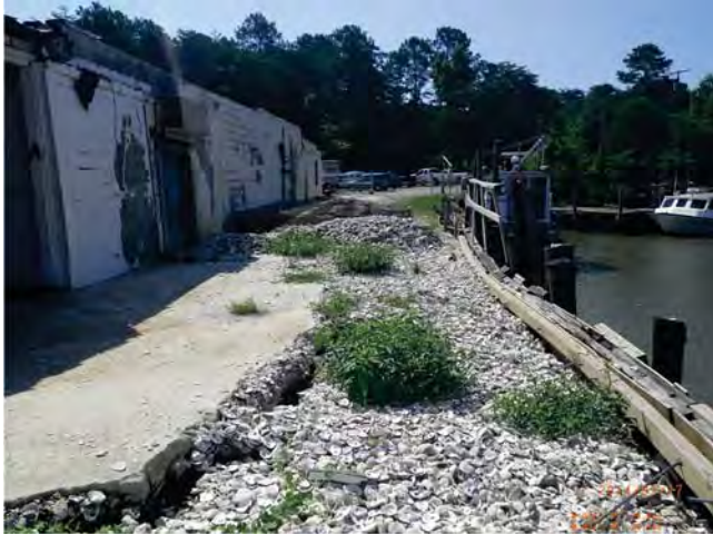
Along one section of the bulkhead, oyster shell has been used to fill in behind the failing structure.
