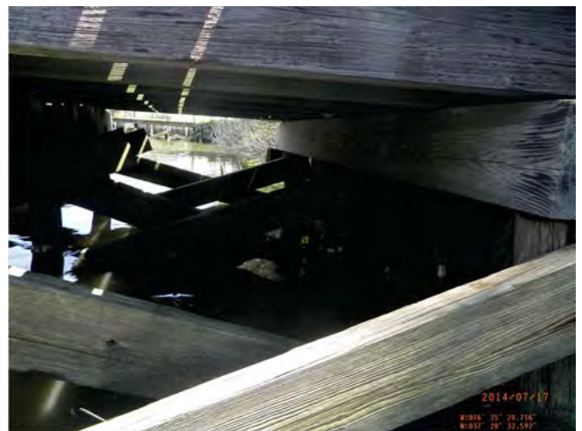
The X braces seem to be intact on the heavy duty section of the dock.
