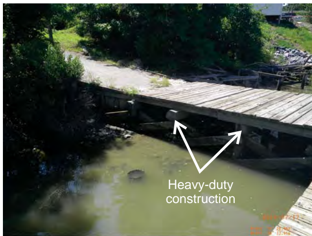
Heavy duty construction consists of 10 in x 10 in cross-beams on the section of pier that is used to load and unload.
