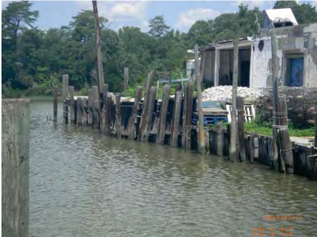
The bulkhead of the private facilities is failing even as minor attempts to stabilize occur.
