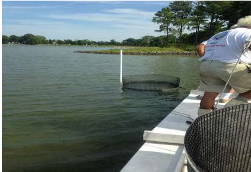
Photo #1: Wire cylinders being installed in Cranes Creek on 08/21/13. Note the filter cloth, just visible above the water. Photo courtesy of Karen Hudson.
