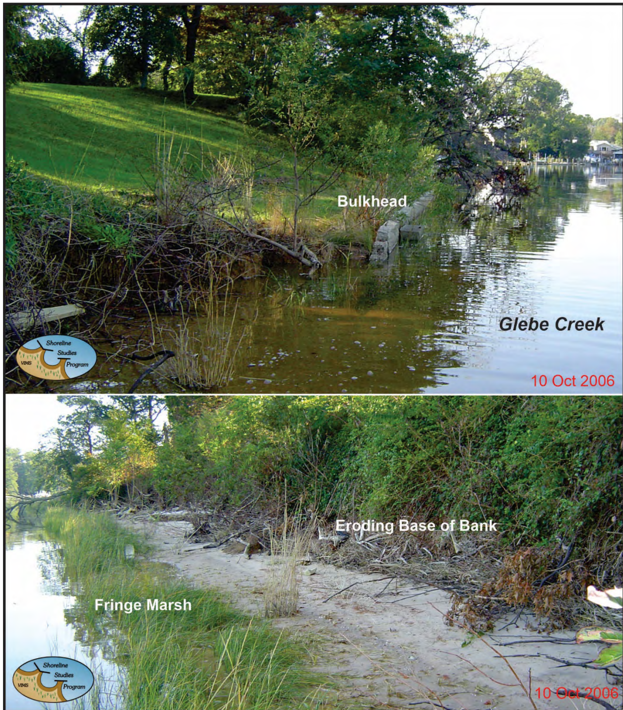
Figure 9-4. Ground photos of the Hull Springs Farm shoreline. Top: the western section of shoreline has a failing bulkhead; Bottom: Post Ernesto: the center section of the peninsula has an eroding base of bank and a fringe marsh. Photo credit: Shoreline Studies Program, VIMS.
